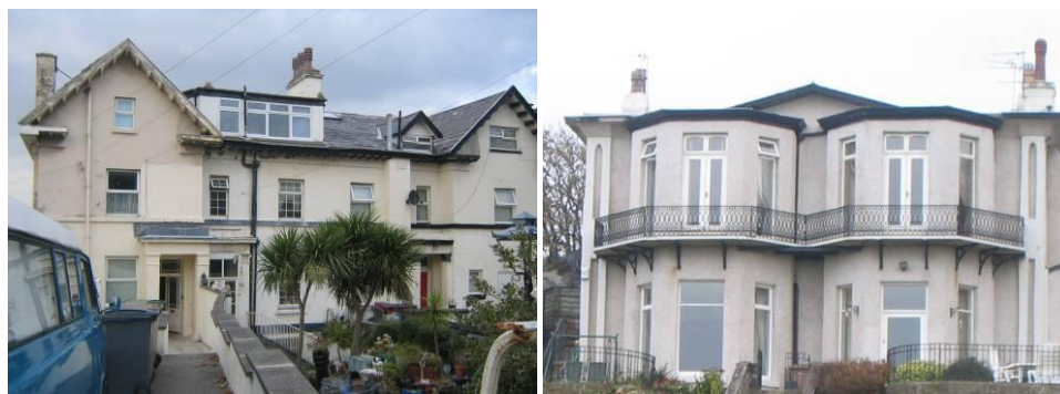
Varied replacement windows, generally diluting the character of the property
